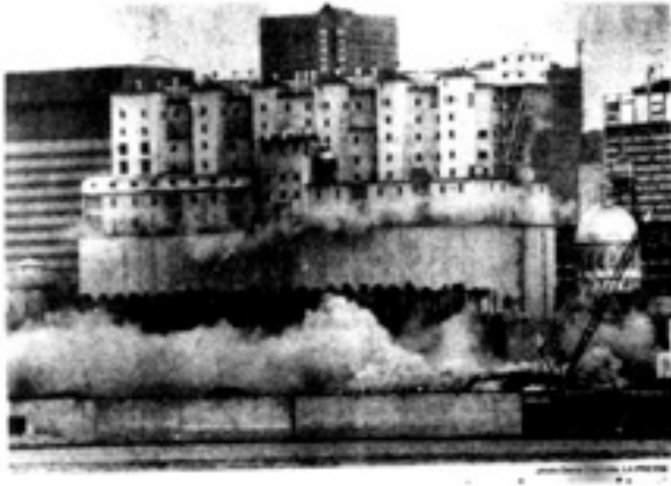
Fig. 9 Demolition of Silo no. 2, as pictured in The Gazette (Montréal), 8 July 1978. CCA Vertical Files, Silo no. 2 .
